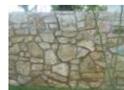
Foundation Damage Due to Drought
